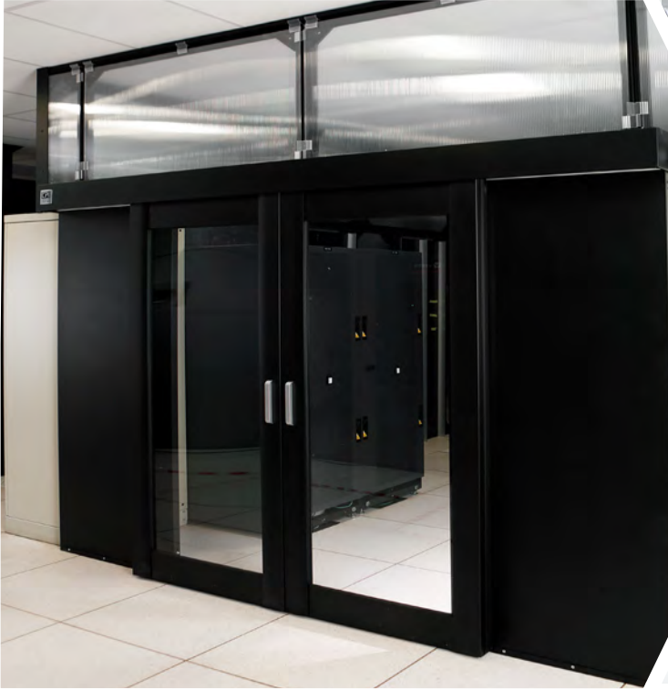
Aisle Containment Isolating hot and cold air in the room
