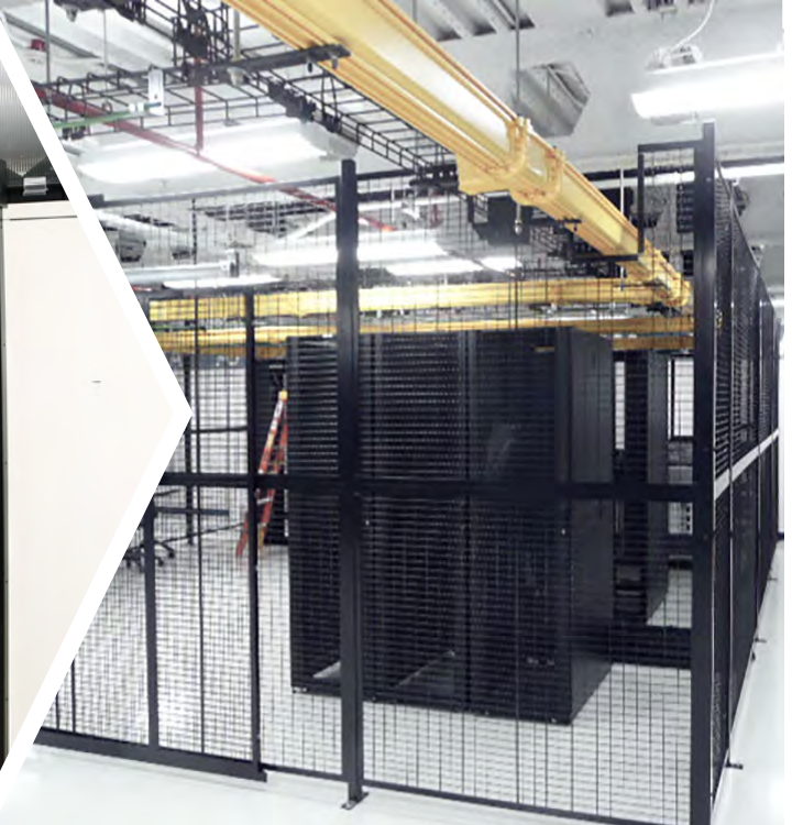
Wire Cage Enclosures Securing equipment in shared spaces
