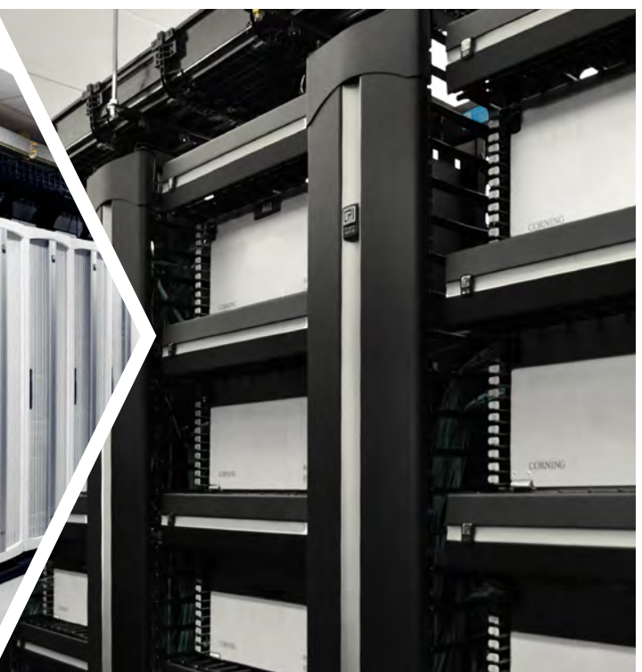
Racks/Cable Management Managing interconnection
