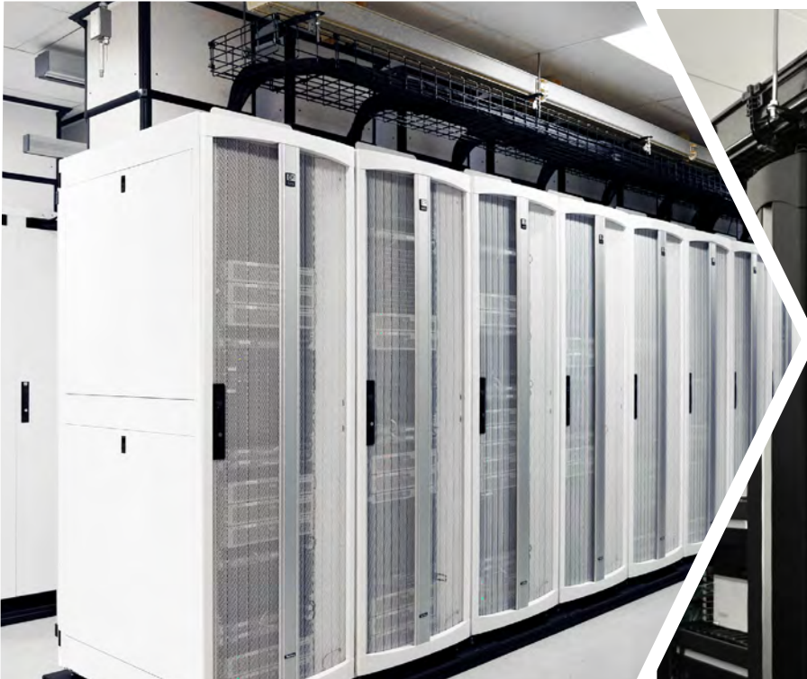
Cable Pathway Connecting equipment in racks
